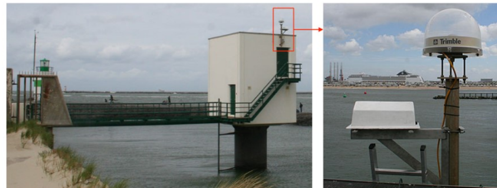
Fig. 1 Example of a collocated transponder-GNSS installation at a tide-gauge in IJmuiden, the Netherlands
